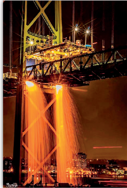
Nightshift ironworkers cutting out a bridge section on the Halifax Bridge. IMPACT funded special welder training for this project.
