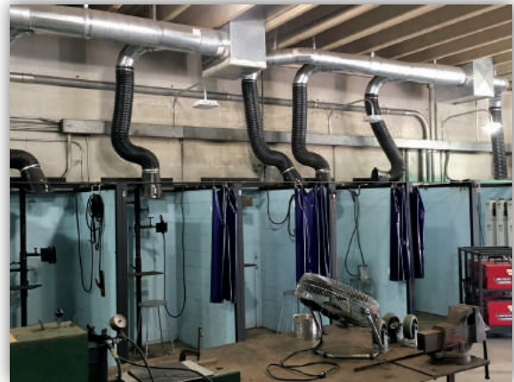
Grant money was used to upgrade the welding shop at the Local 402 (West Palm Beach, Fla.) training facility
