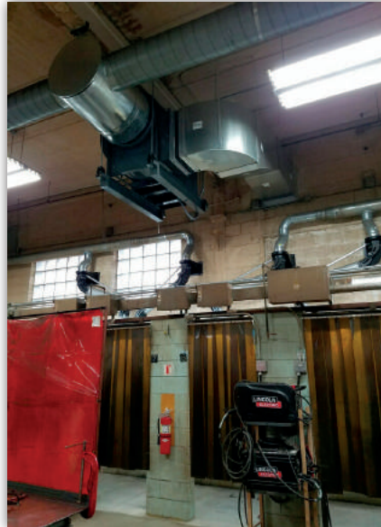
New welding fume extraction system installed in the Local 8 (Milwaukee, Wis.) training facility.
